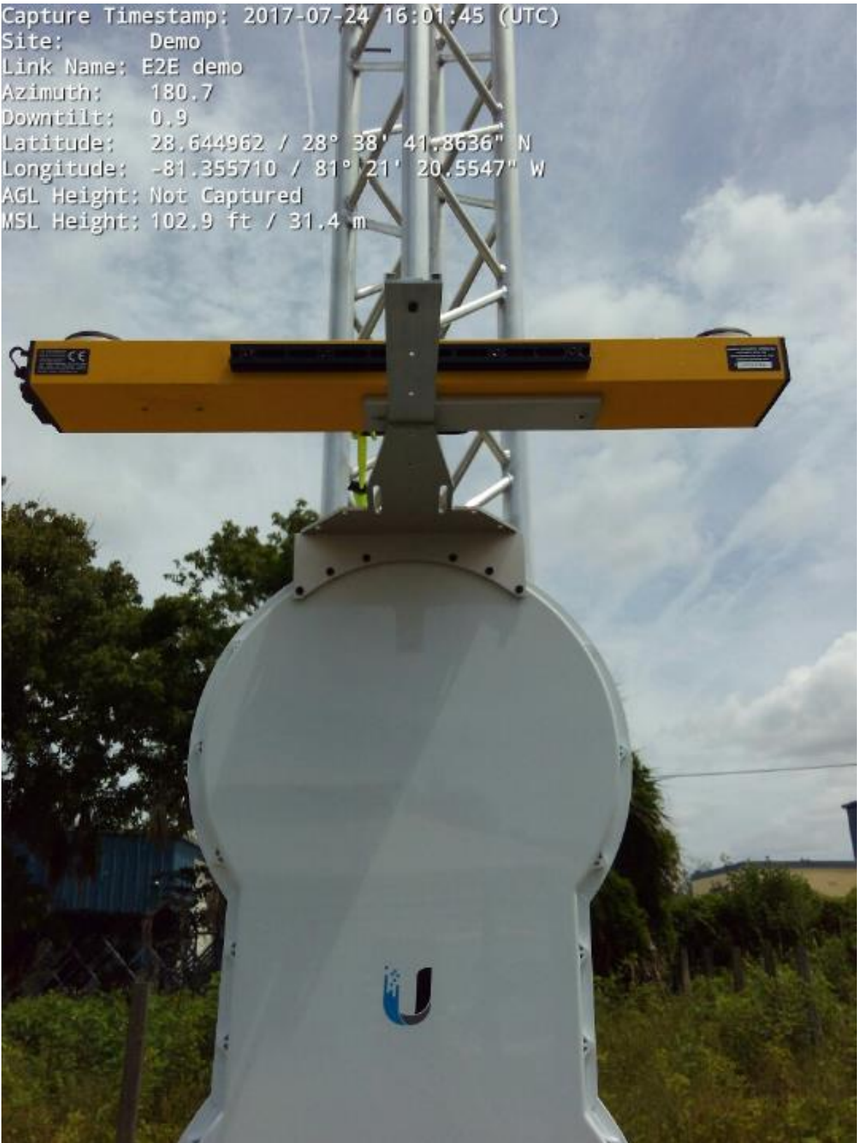
Example End-to-End Microwave Alignment Report with photograph attached
